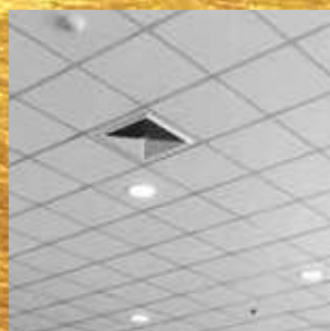
CEILING GRID FALSE CEILING
