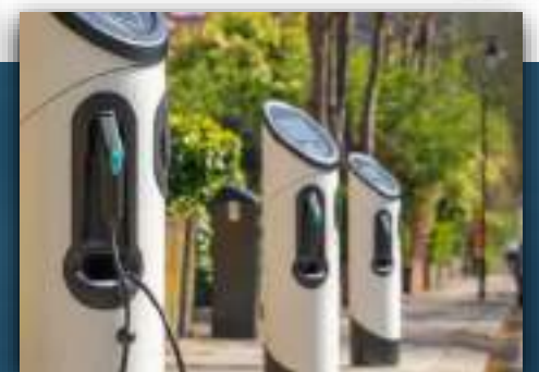
EV Charging Points
