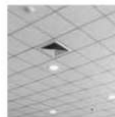
CEILING GRID FALSE CEILING
