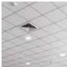
CEILING GRID FALSE CEILING
